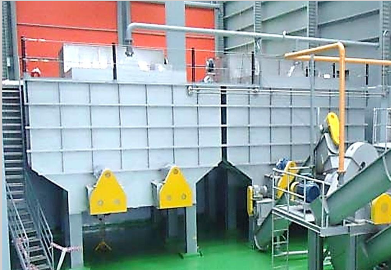
Feed Storage Tank Photo (Reference)
